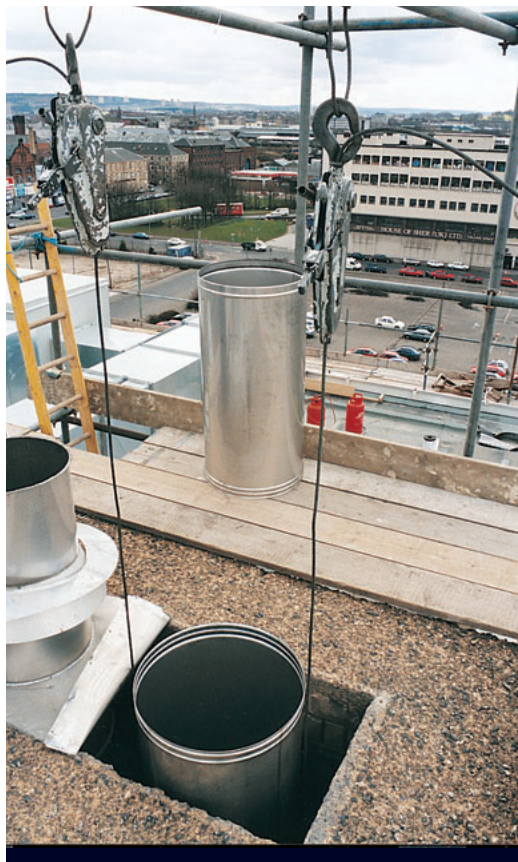
Glasgow Office Complex (see illustration). Supra flue system was used to reline an existing rectangular concrete chimney shaft. The flue was connected to 5 atmospheric gas-fired boilers by QC Gas Vent header sections.
