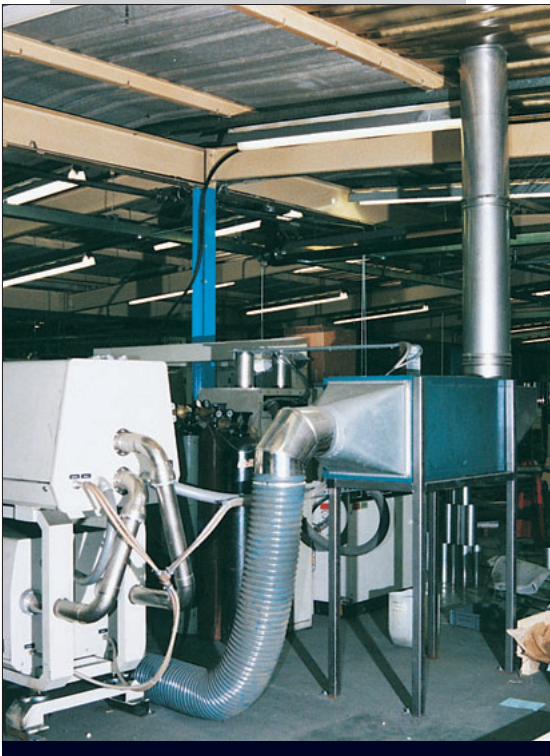
Supra used to vent a particle extraction fan.
