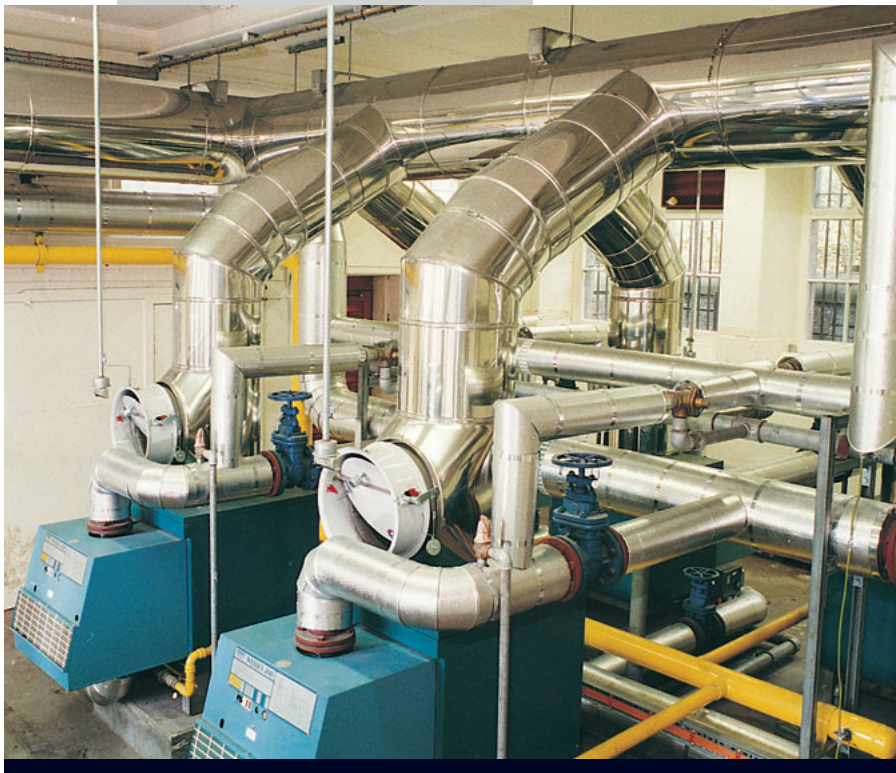
Above Glenogle Swimming Complex, Scotland. SM W chimney and header system serving high efficiency gas boilers.
