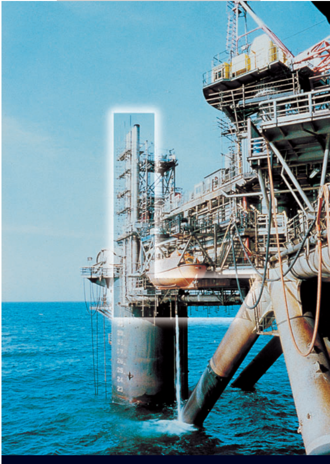
Europa Offshore installed on Talisman Facility's Buchan Platform in the North Sea.
