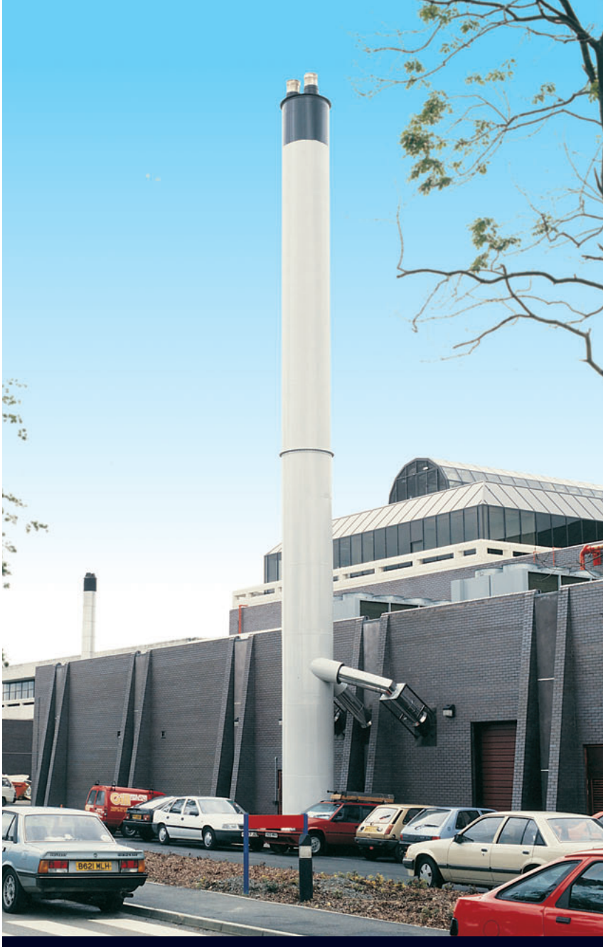
Nationwide Building Society, Northampton. Three Europa Chimney systems installed within a windshield.
